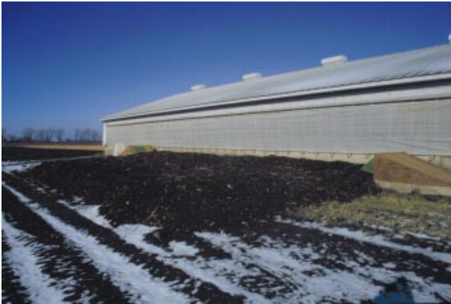
Biofilter on the pit fans of a 1000-head naturally ventilated swine finishing building.
